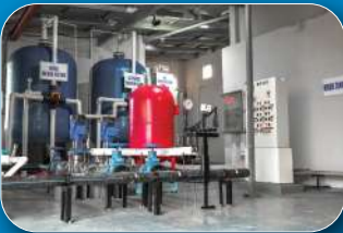
WASTE-WATER TREATMENT PLANTS
