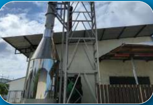
WASTE MANAGEMENT EQUIPMENT
