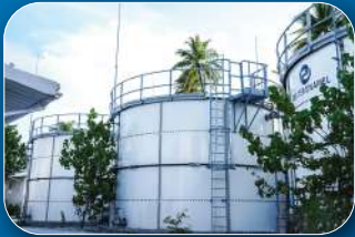
WATER STORAGE TANKS
