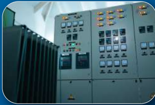
ELECTRICAL DISTRIBUTION BOARDS
